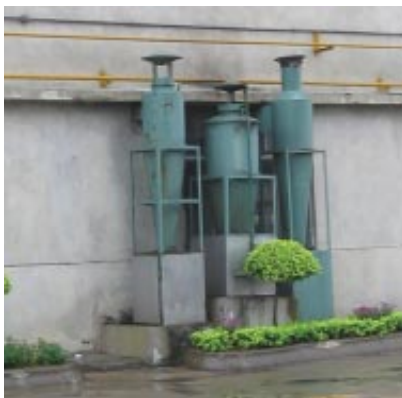
Example of a cyclone in a factory
