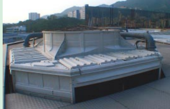
Swire Cooling Towers at Festival Walk – The largest conversion from air-cooled to water cooled air-conditioning plant at that time.
