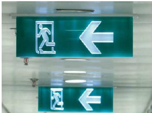
LED Exit Signs
